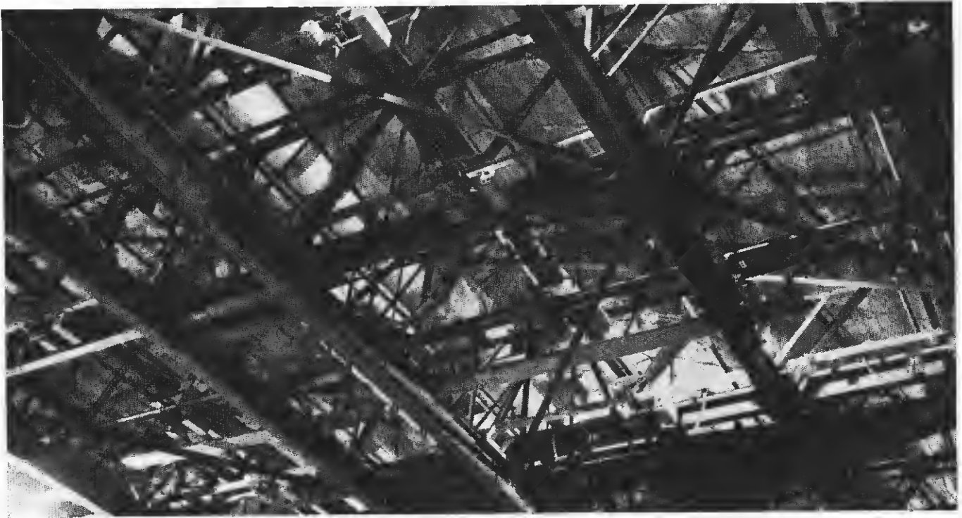
Plate B — Studio 1. Independently supported steelwork incorporating runway beams, motorized lighting batteries, and cable tray supports
